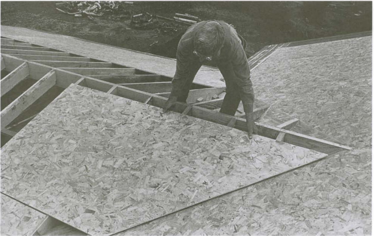
4. Cut along the chalkline and the panel should fit the valley perfectly.
