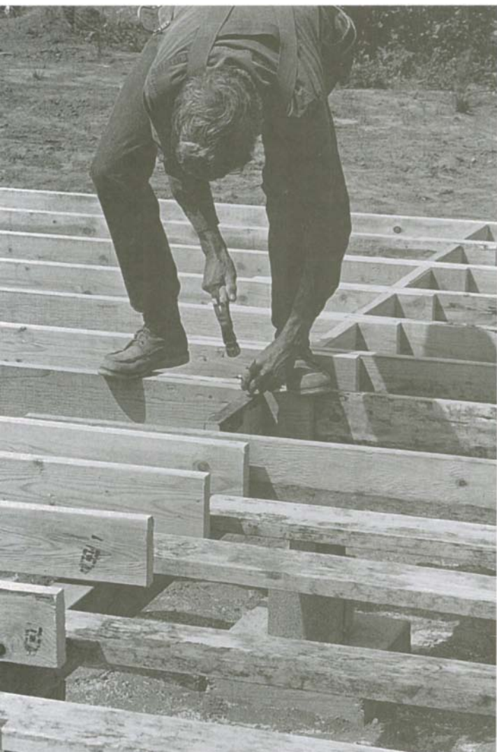
Nail all the blocks and joists in one direction, then turn around and nail from the other side.
