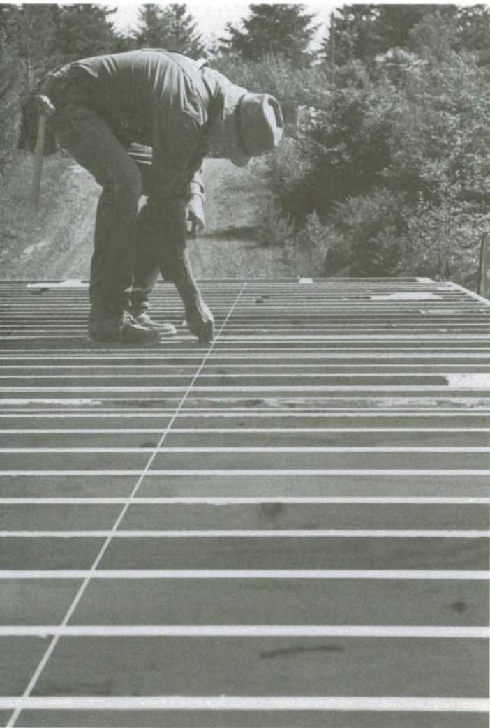
Laying the first row of sheathing to a control line ensures that it will be straight.
