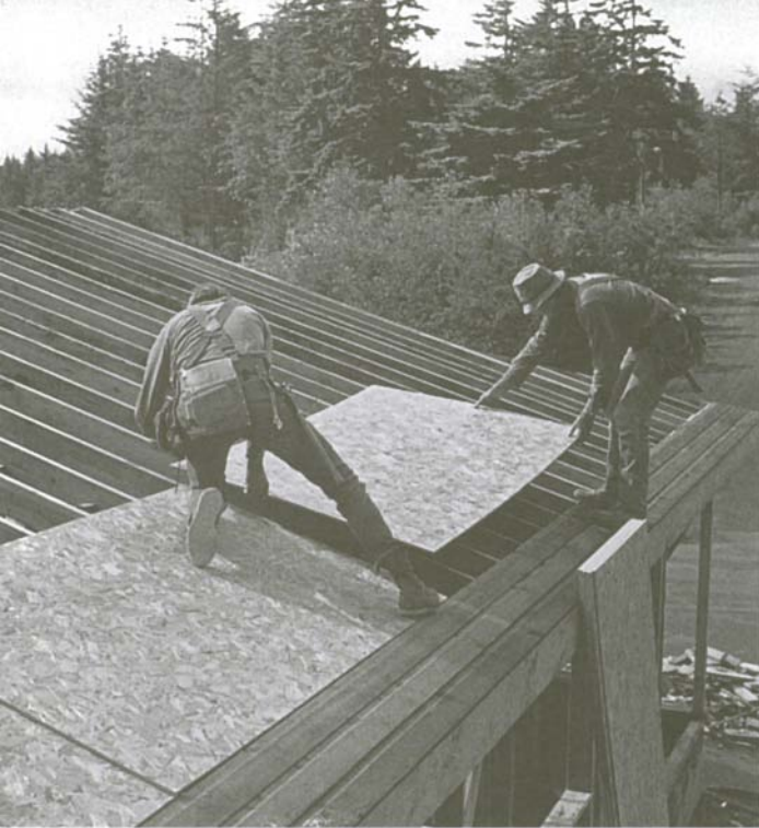
Lay the first course of sheathing along a control line, making sure that the joints break over rafters.
