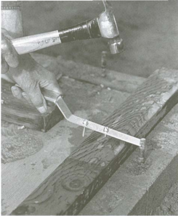
The bottom plate on a slab floor can be marked for the location of anchor-bolt holes using a bolt-hole marker.
