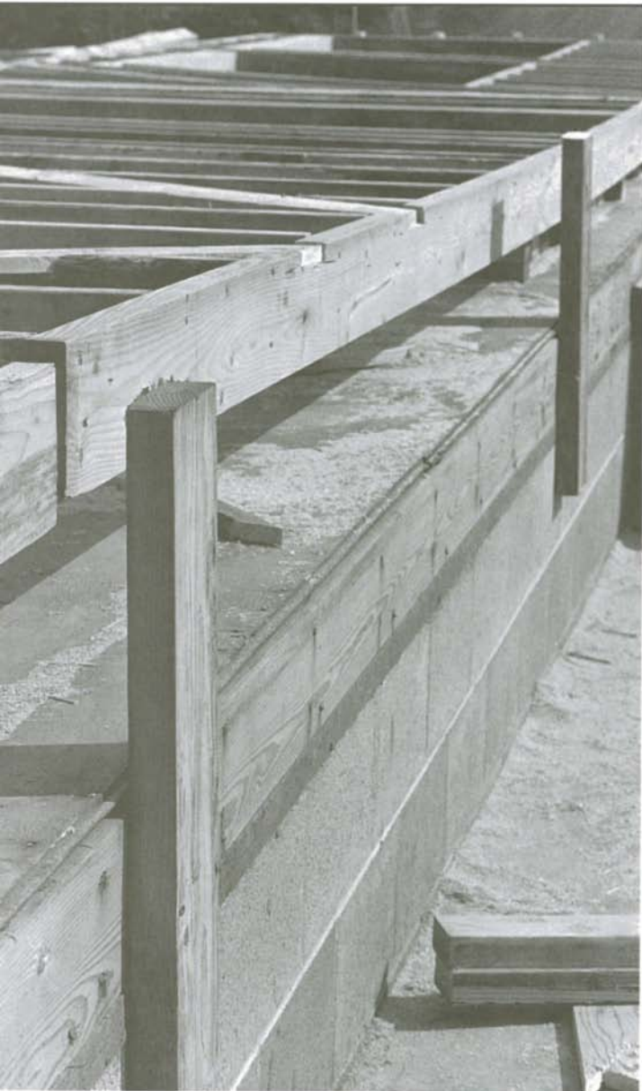
Nail some 2x scraps to the rim joist to keep the wall from sliding over the edge when it's being raised.
