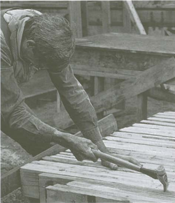
Holding an aligning board in place with your knees, pull the rafters flush using the hammer claws.
