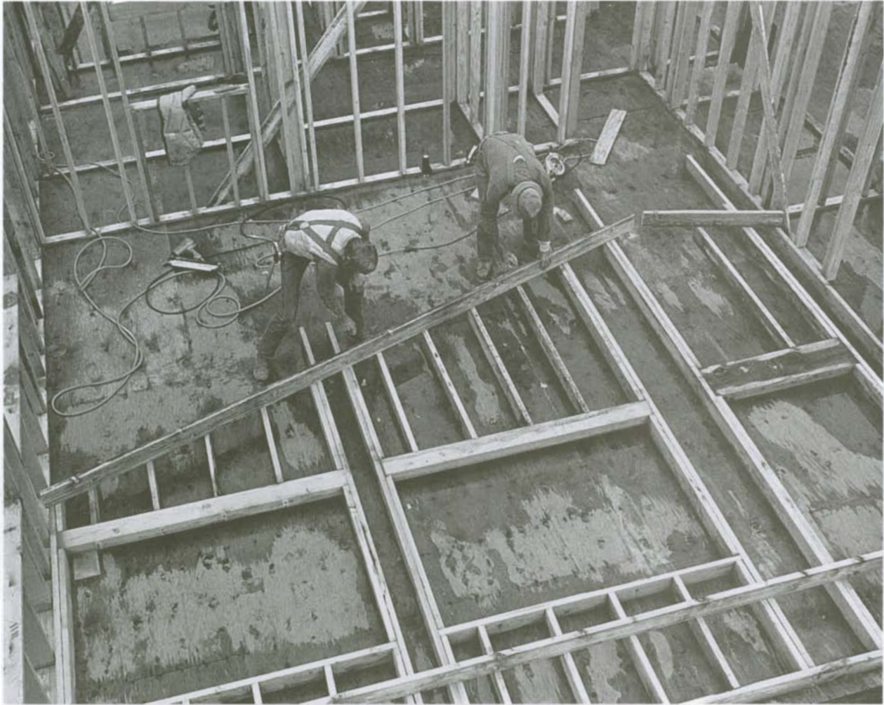
Set the top plate on edge on the chalkline and mark the stud layout on it.
