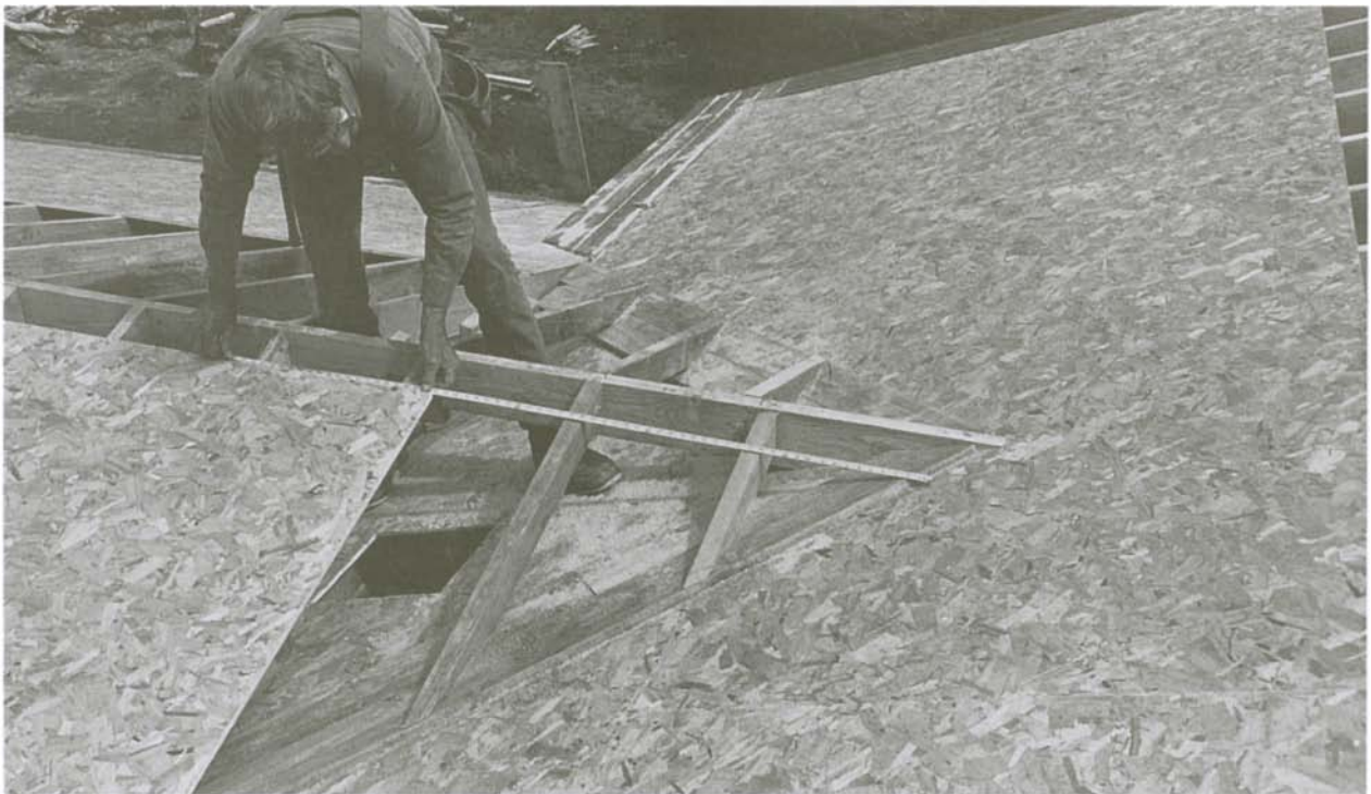
Sheathing a valley: 1. Lay the sheathing panel in place and measure the distance from the upper corner to the valley rafter.
