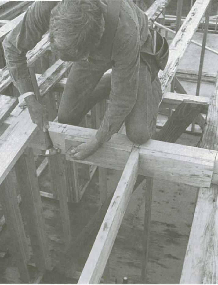
Ceiling joists can be headed off using blocks; floor joists usually require joist hangers.
