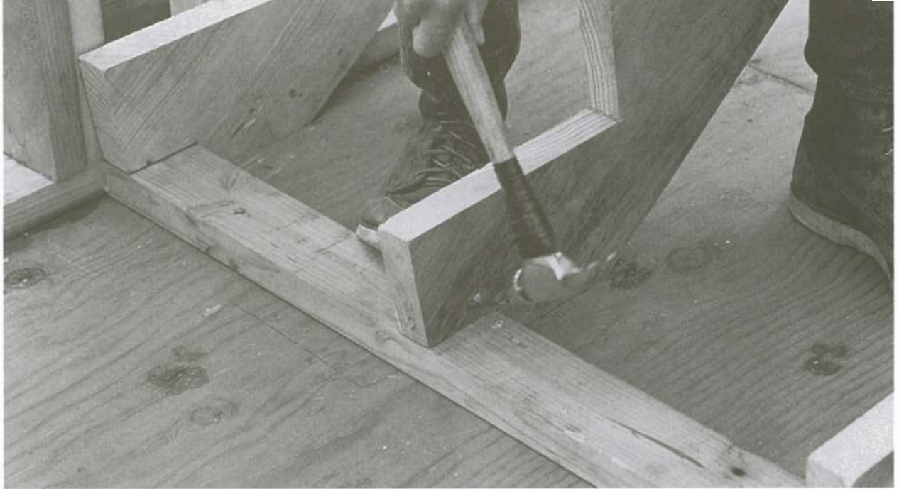
A 2x4 kicker at the bottom of the stairs helps to hold the stringers in place.
