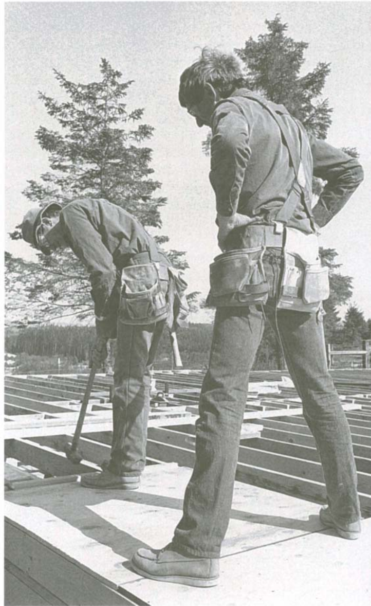
Fitting tongues into grooves sometimes takes extra persuasion. With one person standing on the sheet, another can give it a couple of raps with a sledgehammer. Lay a 2x4 along the edge to protect the groove.
