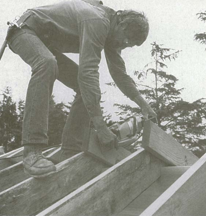
These rafters are resting on a 6x16 beam, which will be exposed in the cathedral ceiling.
