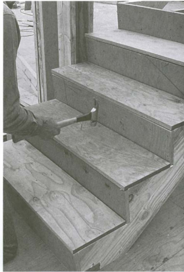
Once the treads have been glued down, secure them to the stringers with 8d nails.
