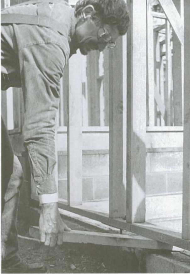
Walls raised on a concrete slab may need to be moved to align the holes in the plate with the anchor bolts.
