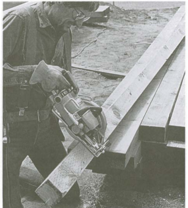
4x4 posts can be cut accurately with a circular saw by keeping the saw table parallel with the edge of the post. Make the first cut and, keeping the saw square, finish by turning the post.
