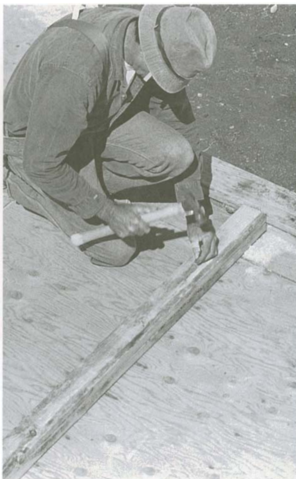
Plates are aligned with the chalkline and then tacked to the floor temporarily with 8d nails.
