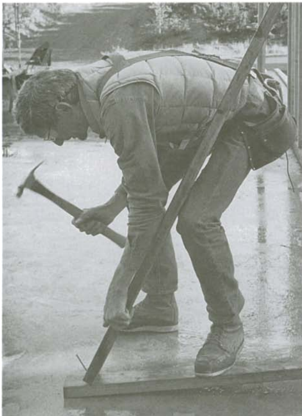
On a concrete slab, nail the bracing stud to a 2x nailer secured to the bottom plate.
