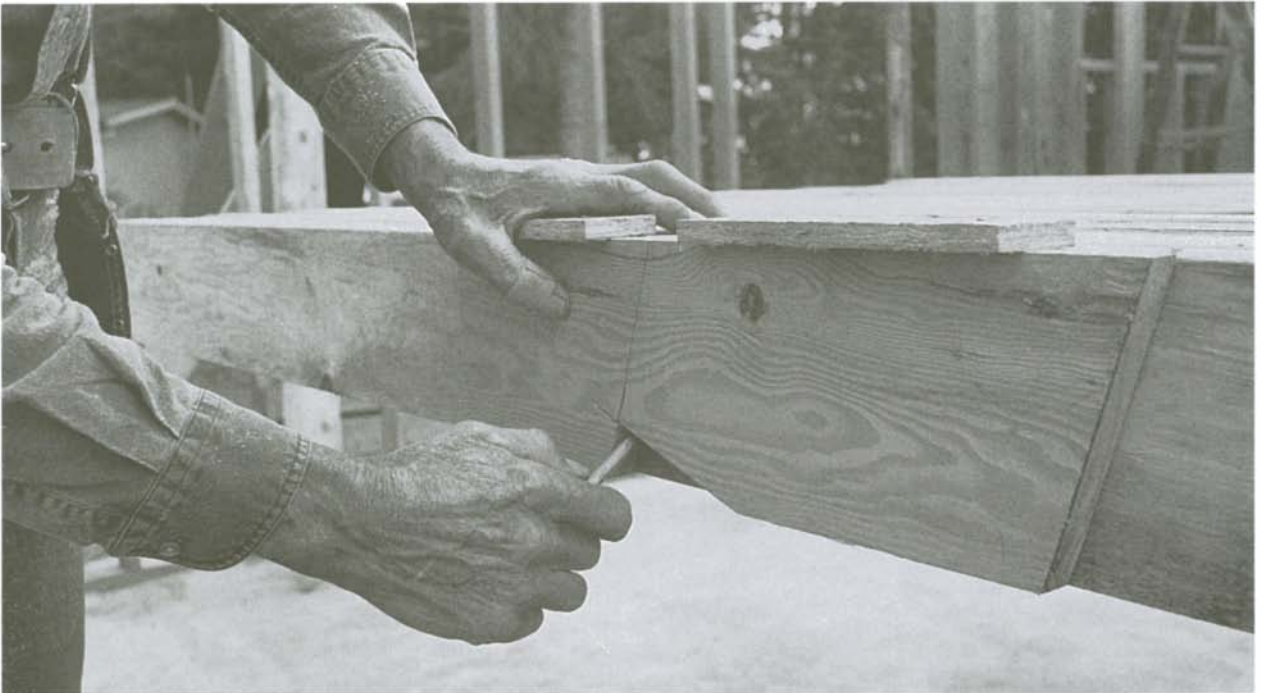
Use the same template to mark the bird's mouth. Match the registration mark on the template with the chalkline on the top edge of the rafter.
