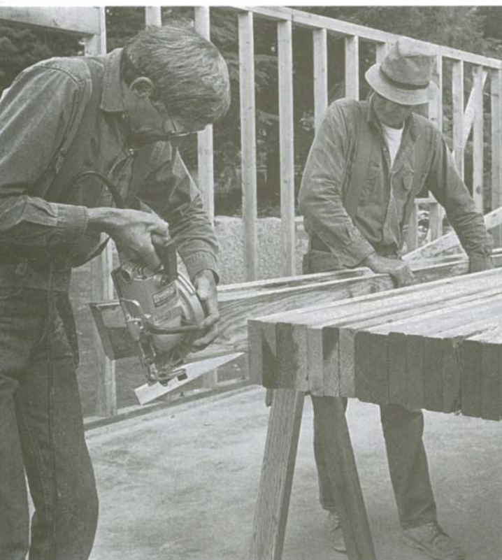
Once all the rafters have been marked, make all the ridge cuts.
