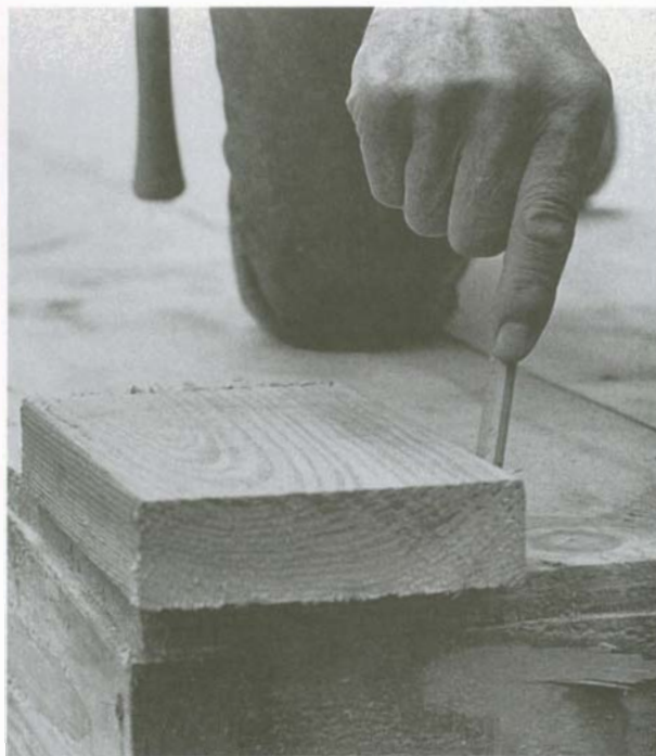
The locations for outside wall plates can be marked using a scrap piece of plate stock as a guide. Make sure to hold it flush with the edge before marking. Do this at both ends, then snap a chalkline between the two marks.
