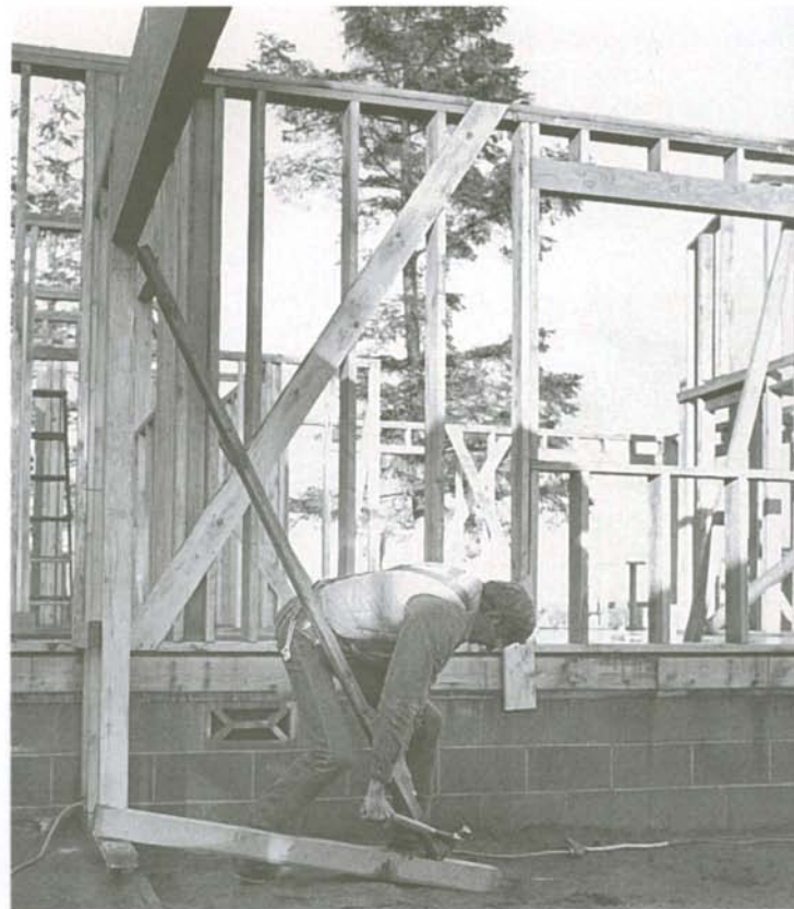
At ground level, walls can be pushed in and braced by nailing a 2x to the bottom plate and running it out from the building, providing a nailing surface for the brace.
