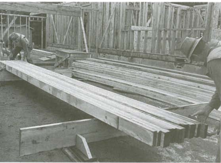
Simple site-built rafter horses allow you to mark and cut all of the common rafters at once.
