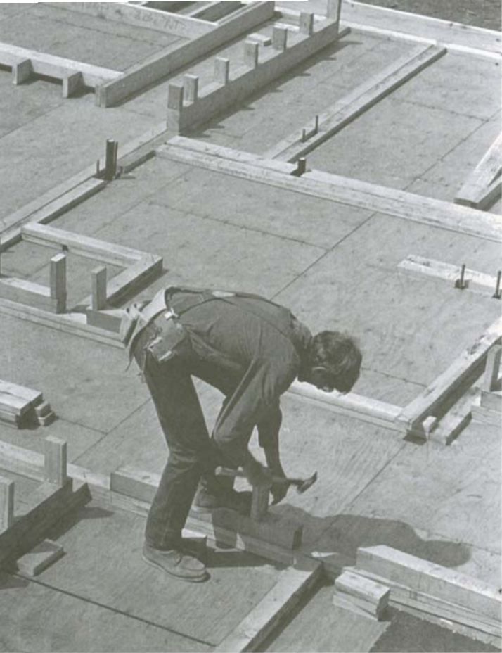
Nail all the cripples to the headers and rough sills before building the rest of the walls.
