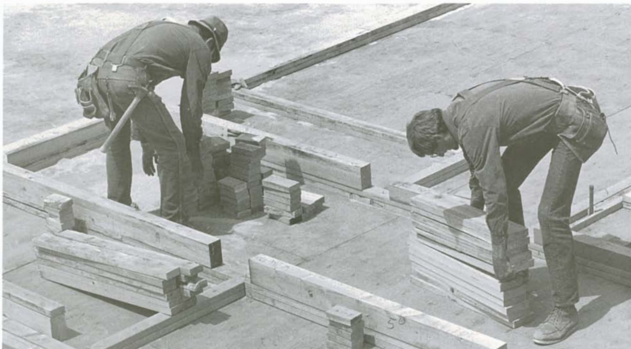
Scatter all top and bottom cripples to their respective door and window headers before beginning to nail them on.
