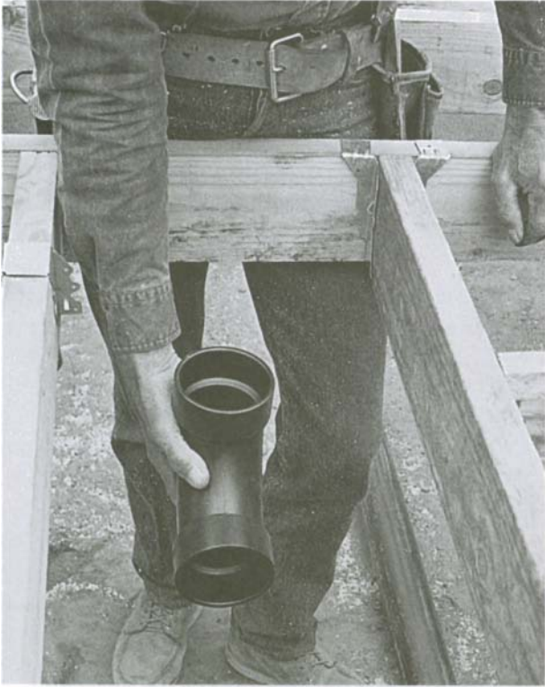
This opening, or 'headout,' in the floor has been framed in to allow for plumbing for a toilet.
