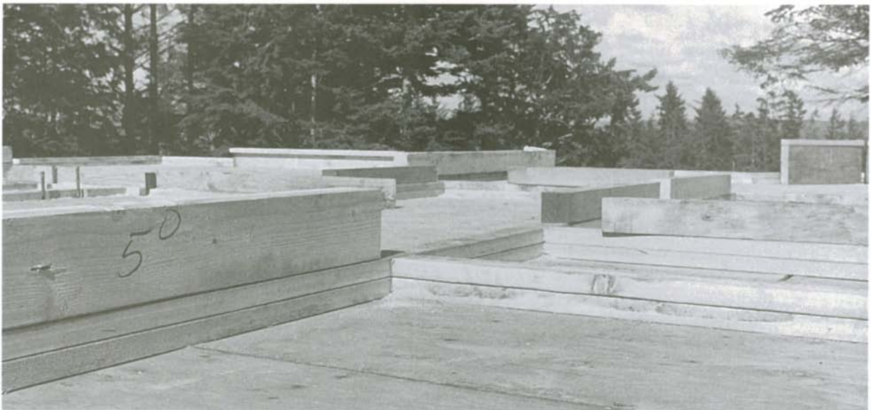
Place each header on the plates, near its location in the wall frame.
