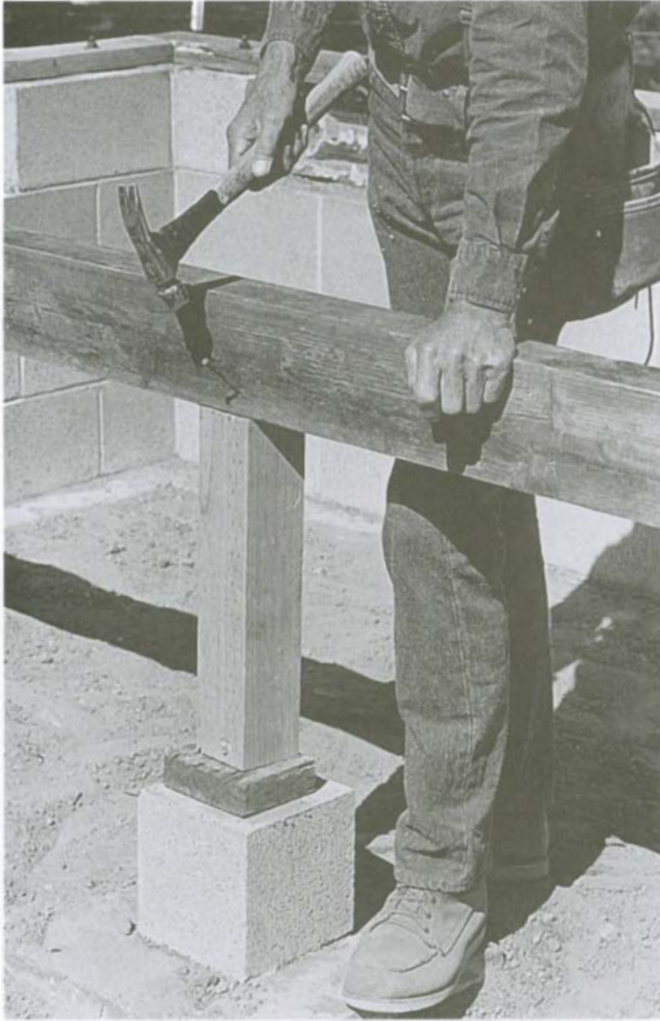
Girders are nailed securely to each post with three 16d nails or four 8d nails, helping to tie the entire frame to the foundation.
